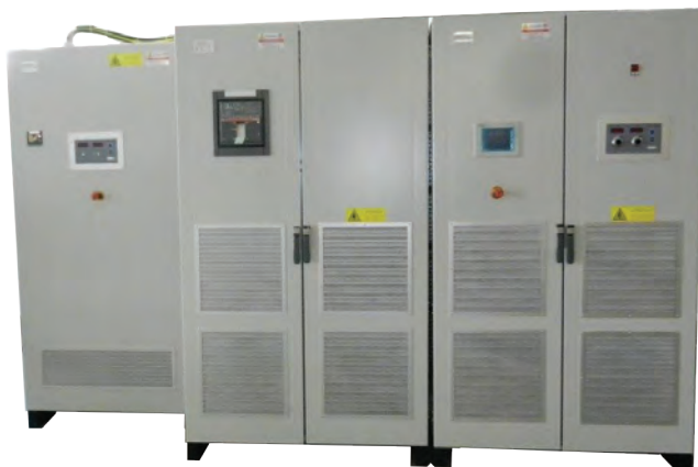
Example of an AL3000R unit rated at 500kW
